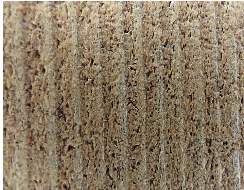
Penetrating Stain – Some surface fungi growth Note different stain penetration (with some residual on surface) between late and early wood grain Coating no longer hydrophobic
